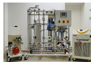
Pilot filtration plant.
